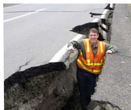
Prof. Kyle Rollins (BYU Civil Engineering Dept.) in a fissure formed by failure of roadway over soft ground.
