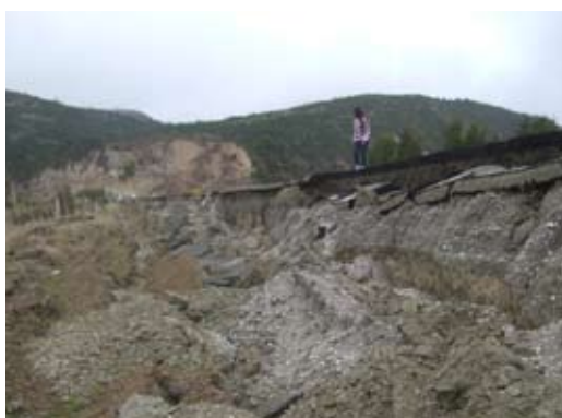
Failure of highway embankment over soft ground in Magnitude 8.8 Chilean earthquake.
